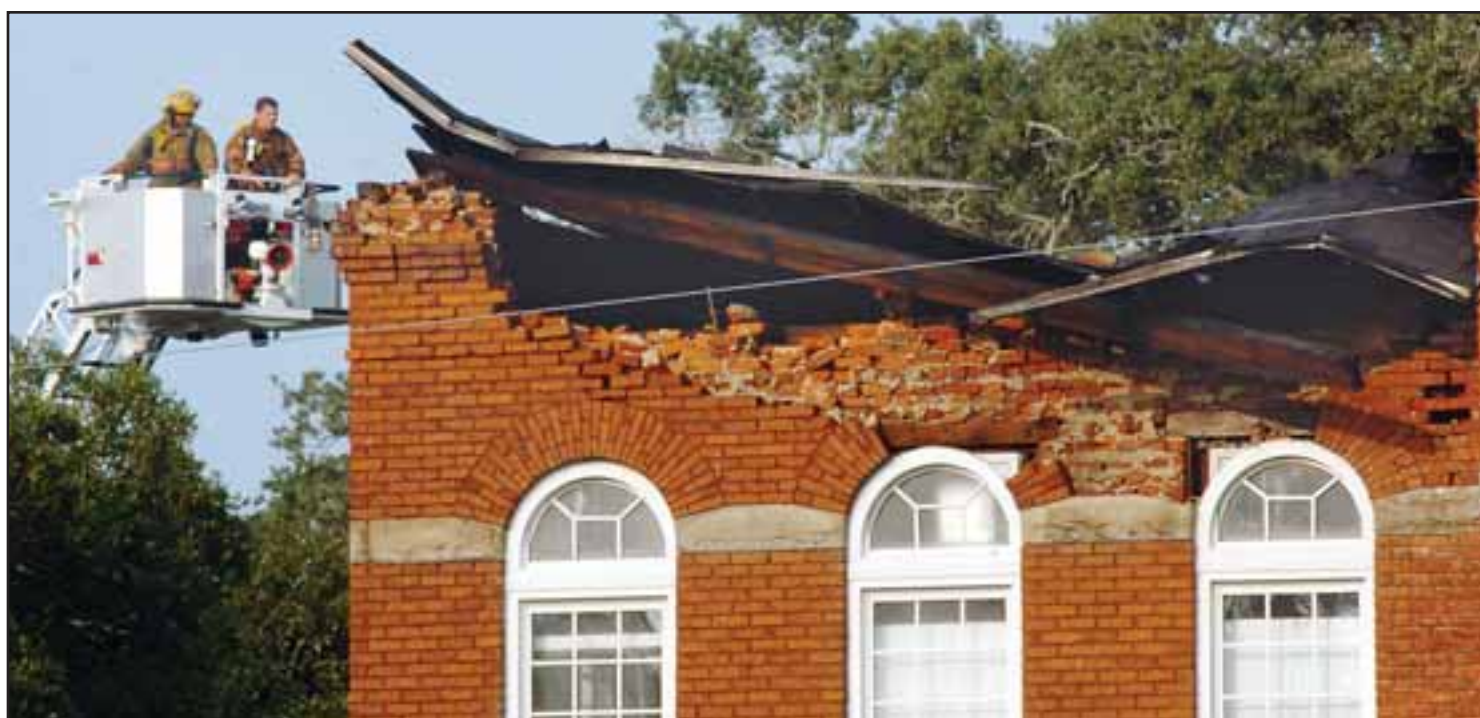
Firefighters rise above the Glynn Academy Annex at about 9 a.m. Friday to survey fire damage. Bobby Haven/The Brunswick News
